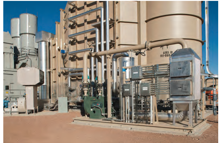
Ammonia skid-SCR system
