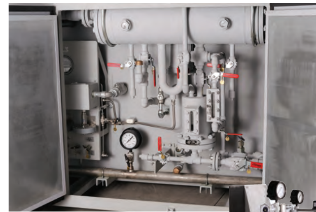
Fluid system sub assembly with piping, vessels and instruments.
