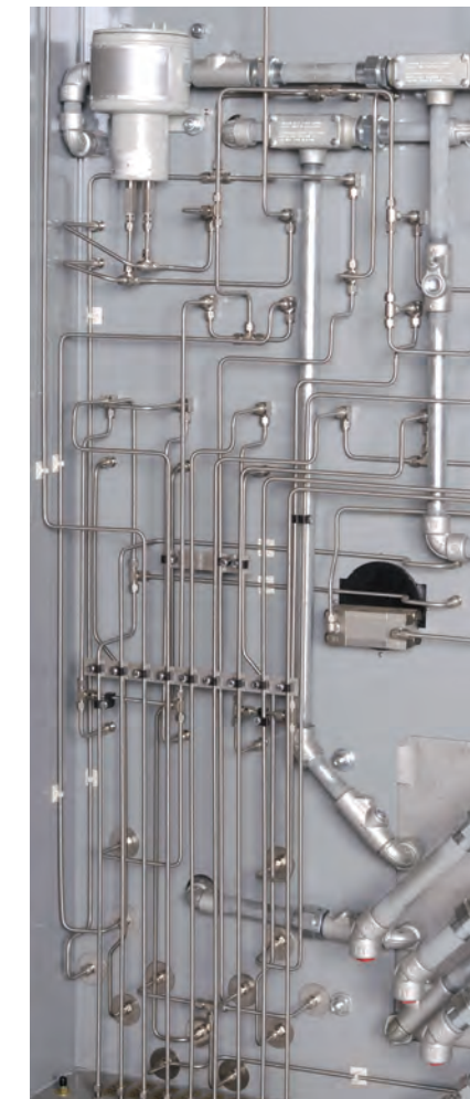
Hydrogen Monitoring Panel
